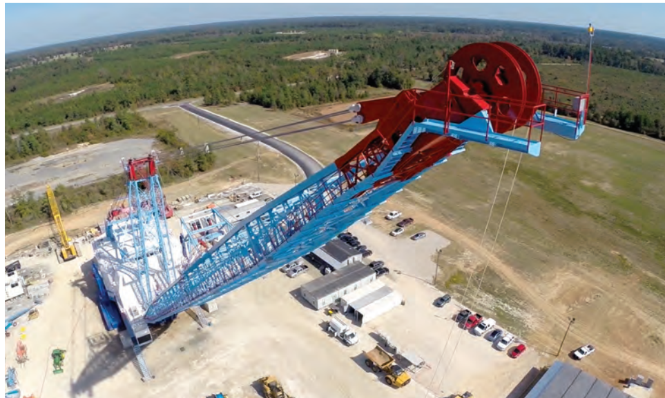
The dragline features a 57-ft diameter roller circle and a 320-ft boom with a 290-ft operating radius at a 38° angle.
